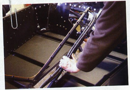
Running supply and return fuel feeds through centre tunnel.
