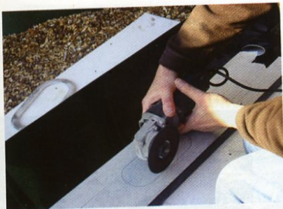
Using an angle grinder for exhaust outlets in the side panel. Carefully does it!
